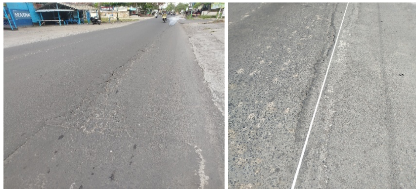
Figure 5. Moderately Damaged Condition
