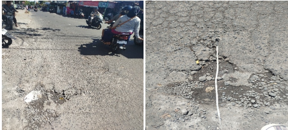
Figure 4. Condition of Minor Damage
