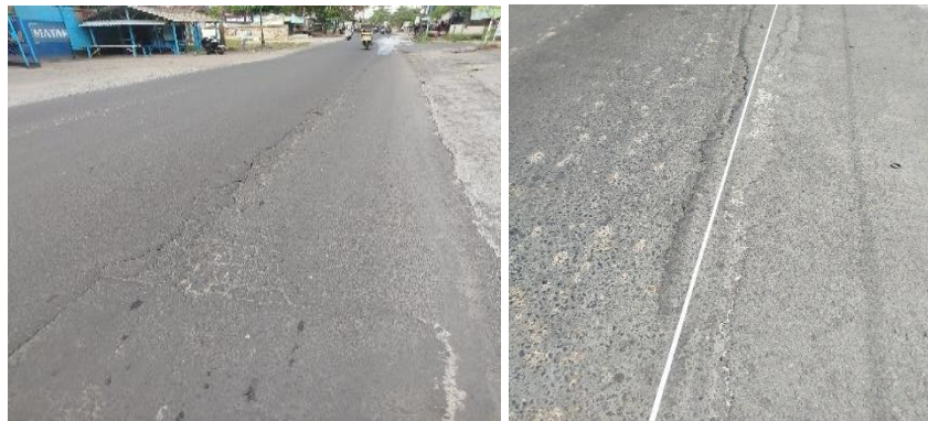
Figure 5. Moderately Damaged Condition
