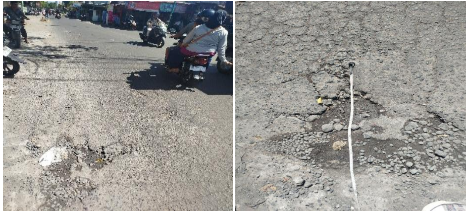
Figure 4. Condition of Minor Damage
